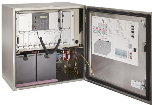
Figure 2: Electronic Siren Control Panel
