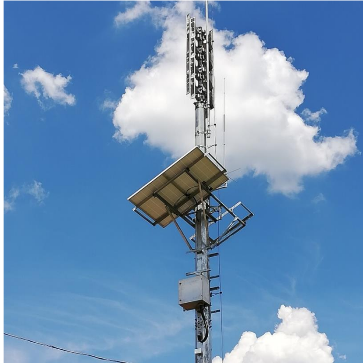
Figure 4: Electronic siren with solar power
